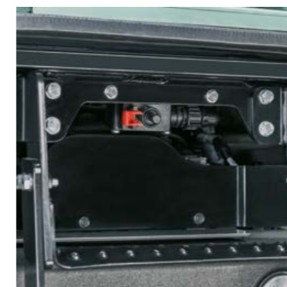
The battery isolating switch is conveniently located on the left access step
